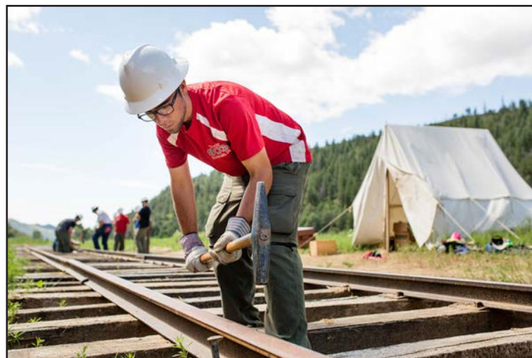
Eric Longoria from Troop 803 of Hockenessin, Delaware works on the railroad at Metcalf Station on Wednesday, July 15. Crews that work on the railroad have to move four 250 pound rail ties before they can begin to set spikes into the track.
