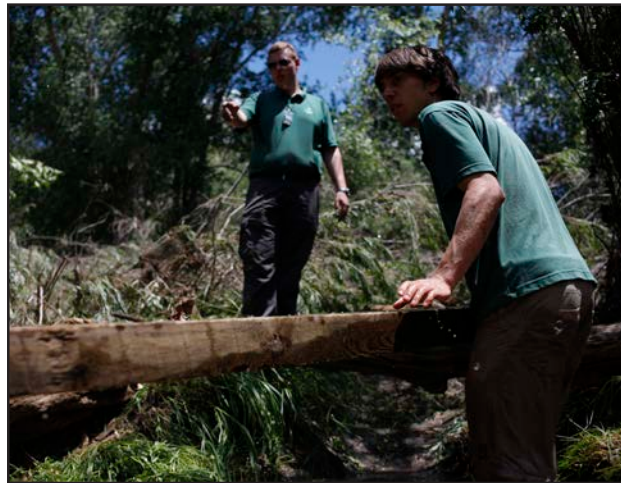
Nicolai Johansen, an international staff member from Denmark, directs Chris Heden, CD of Indian Writings, where to place the new bridge. Heden, Johansen and other staff spent a major part of the day after the flood replacing bridges that were destroyed in the disaster. Josh Galemore/Philnews
