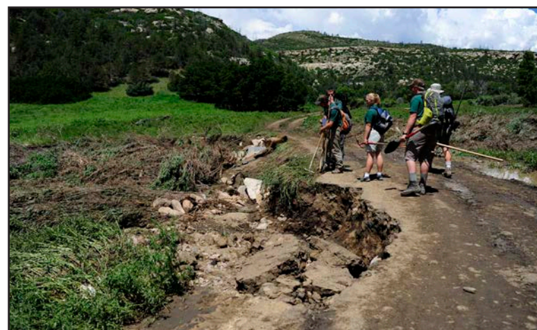
Top photo: Flood water washed away part of the road during the 1965 flood. Below: 2015 flash floods washed away part of the road to Indian Writings. Justin Gilliland/PhilNews
