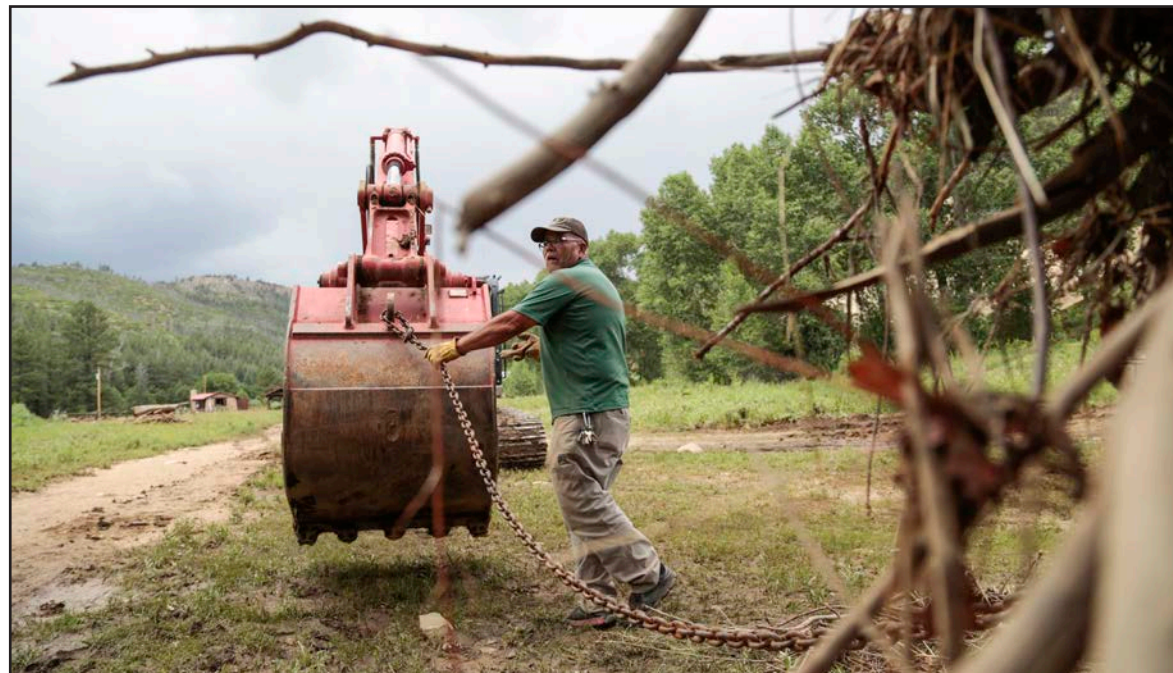
Leo Martinez secures a chain between a backhoe and a large metal grill basin which was washed downriver from the Ponil Chuckwagon area and deposited in a debris pile during the flash flood of June 27. Martinez said he had never seen flooding of this magnitude in decades of living in Cimarron. Leanora Benkato/PhilNews
