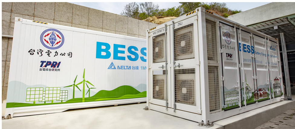
Delta built Taipower's largest energy storage system at Xia Xing Branch Power Station of Kinmen Tashan Power Plant.
