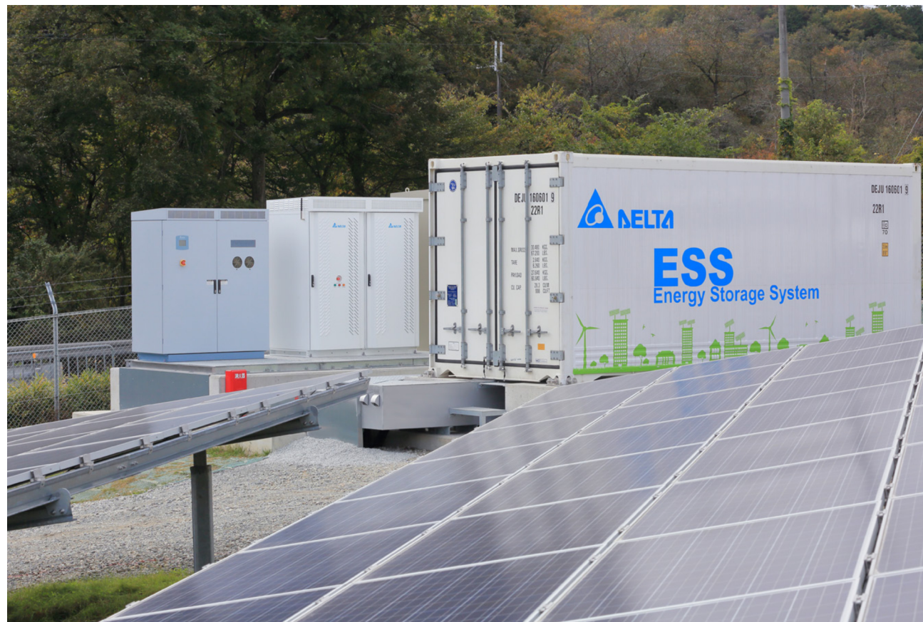
Delta's Energy Storage Solutions
