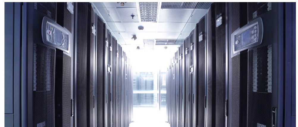
Delta created the first Uptime Tier III TCCF (Tier Certification of Constructed Facility) data center in Vietnam for Hanoi Telecom's subsidiary company HTC-ITC.
